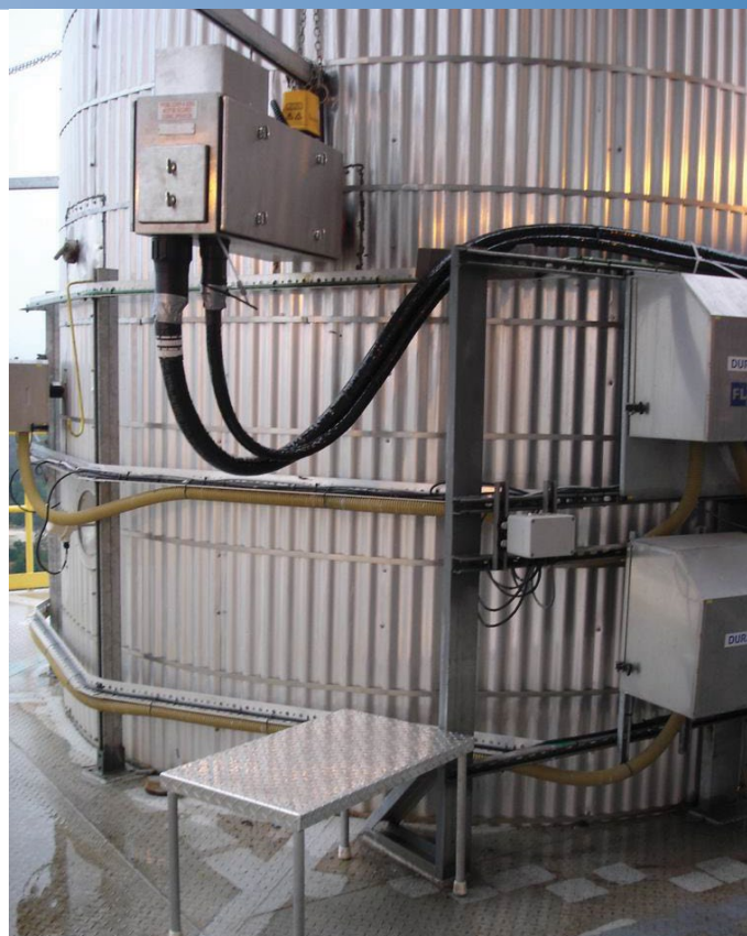
Figure 1: View of the Model 83i Probe at southeastern cement kiln.
